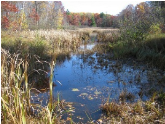
Downstream of NN culverts with backed up water from downstream beaver dams on Osprey Creek.
