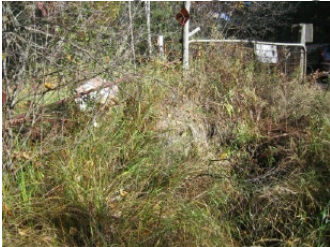
Downstream of Thunderbird Road driveway with virtually no water getting through the present obstruction.
