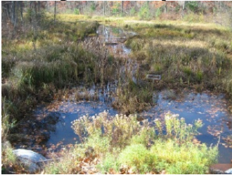
Culverts downstream side of NN with standing water from backup caused by 7+ beaver dams downstream.
