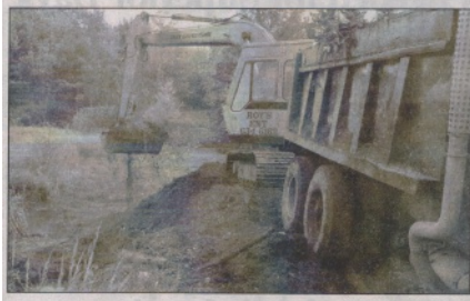
Submitted by Tom Burgess A Roy's Enterprises excavator removes dirt fill from a wetland and Osprey Creek where Snowmobile Trail Three crosses it. The creek restoration project was done last week to allow a pond created by the obstruction to drain.
