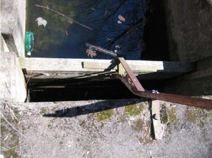
Placid Diversion Canal Dam looking down on boards which are held and locked in with
